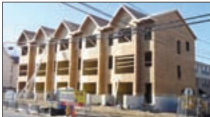
The City of Wilmington transferred a large parcel of land to WHPartnership that was once the site of the Jimmy Jenkins Center. Construction has begun on the 9 unit, townhome development that will receive LEED Silver certification.
